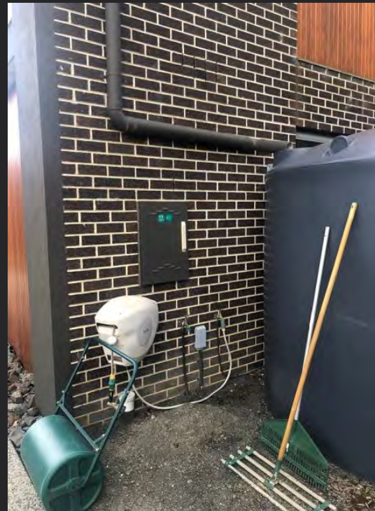
Switchboard in relation to the garage
