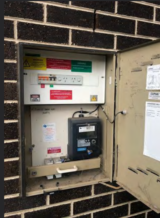
Switchboard Close Up
